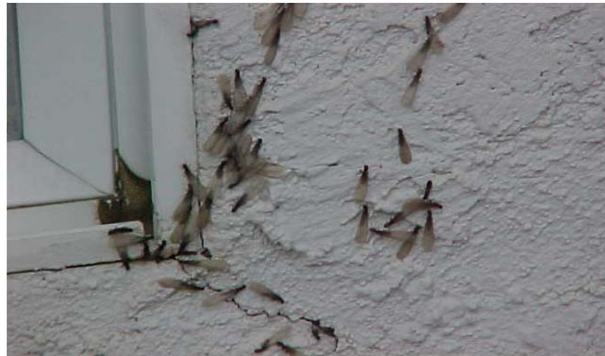
Termite swarmers on the wall of a home.
