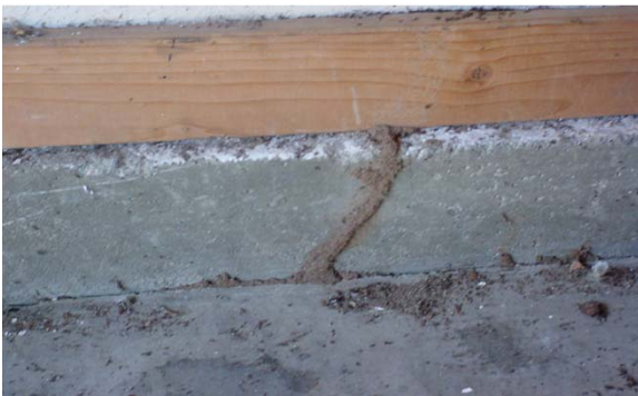
Termite Tube bridging a garage slab expansion joint and entering the wall framing.
